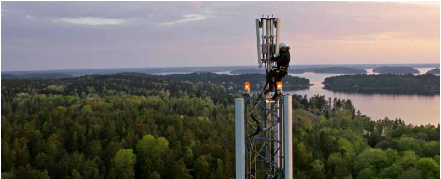
Following our Zero Tolerance Safety rules and proper training are crucial both for employees and suppliers working in high risk environment.
